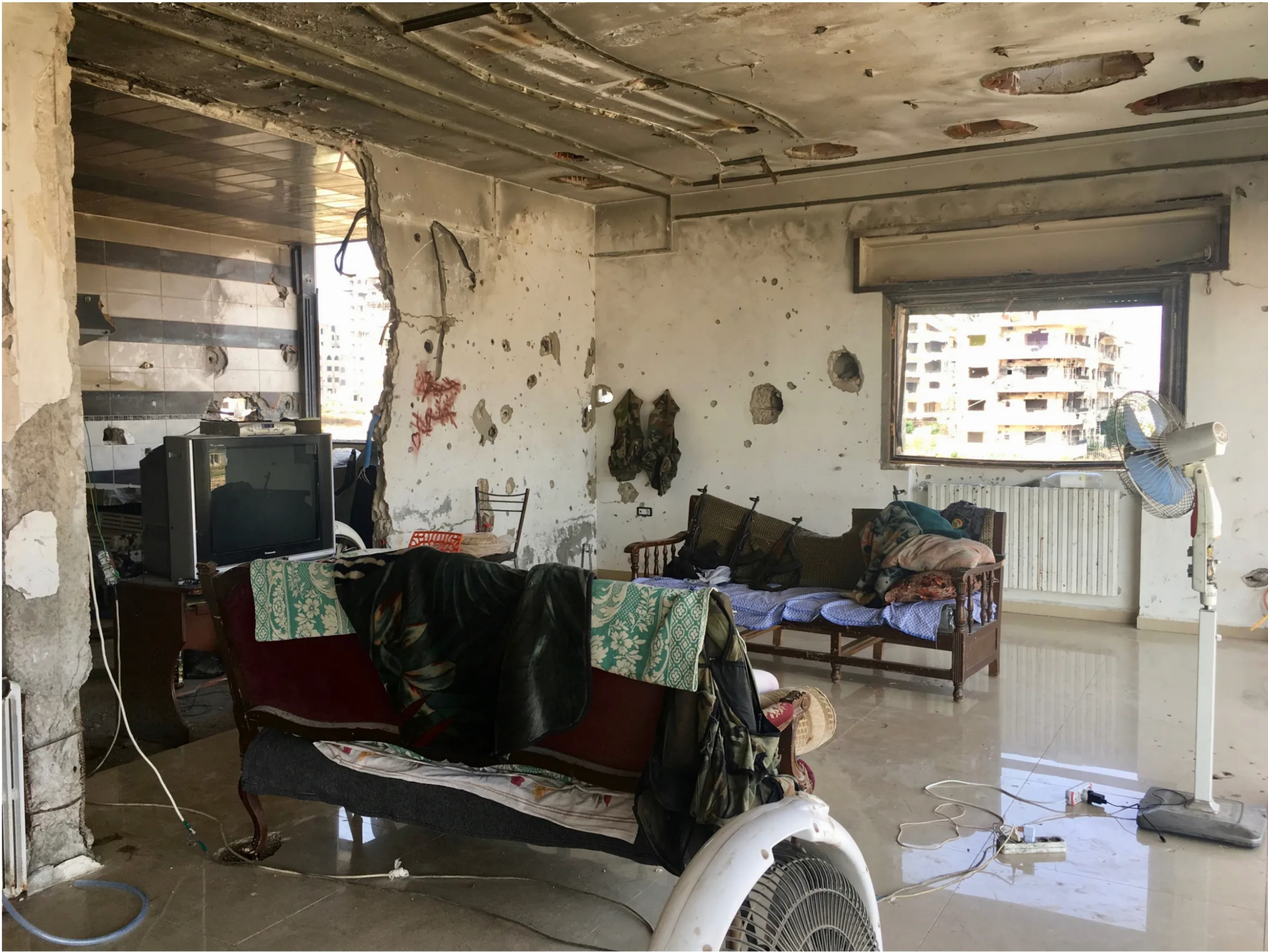
Destroyed apartment in Waer being used as a post by Syrian security.
